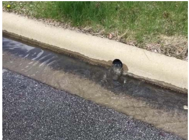
Incorrect Sump Pump Discharge
