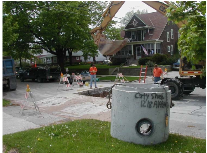
Precast Manhole with Rubber Boot
