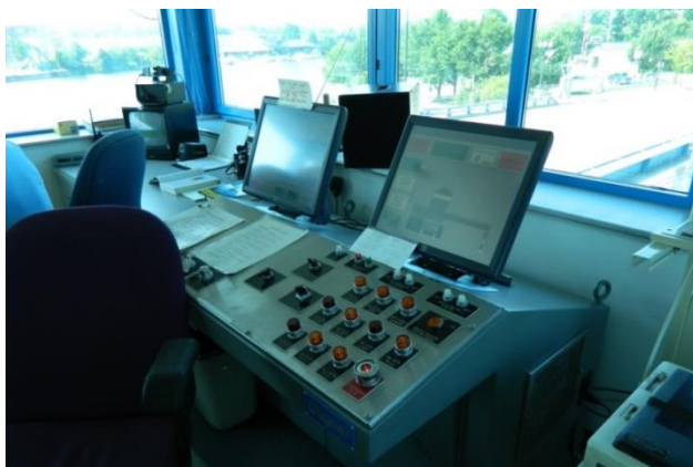
8th Street Bridge controls
