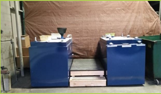
OIL COLLECTION TANKS
