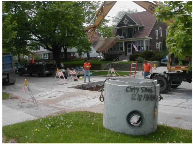
Precast Manhole with Rubber Boot
