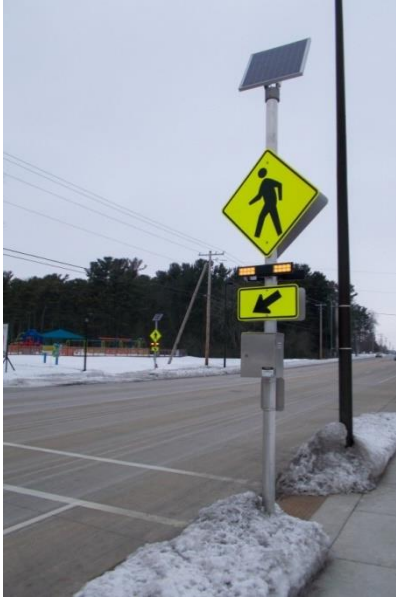
RFB System near Shaw Family Playground
