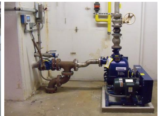
New Scum Pump for Final Clarifiers #1 and #3
