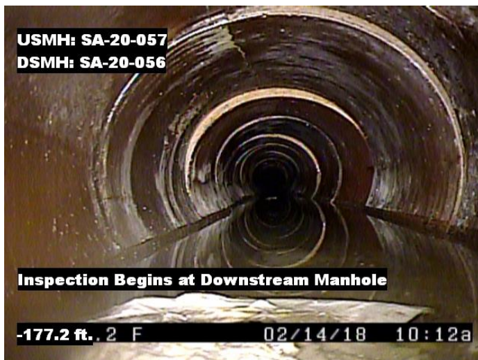
Debris in a Sanitary Sewer
