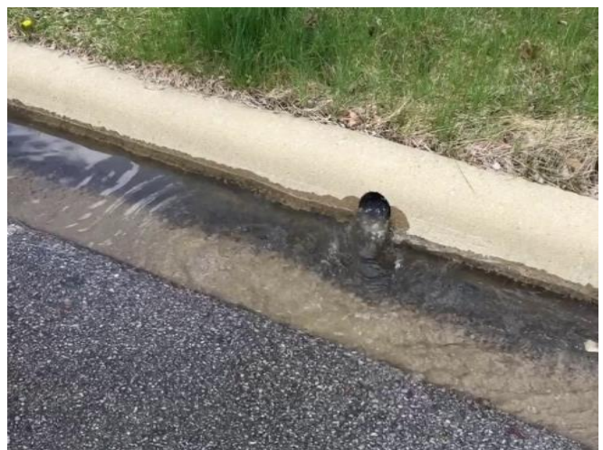
Incorrect Sump Pump Discharge
